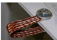
Ground Wire Grounding wire Between panels
